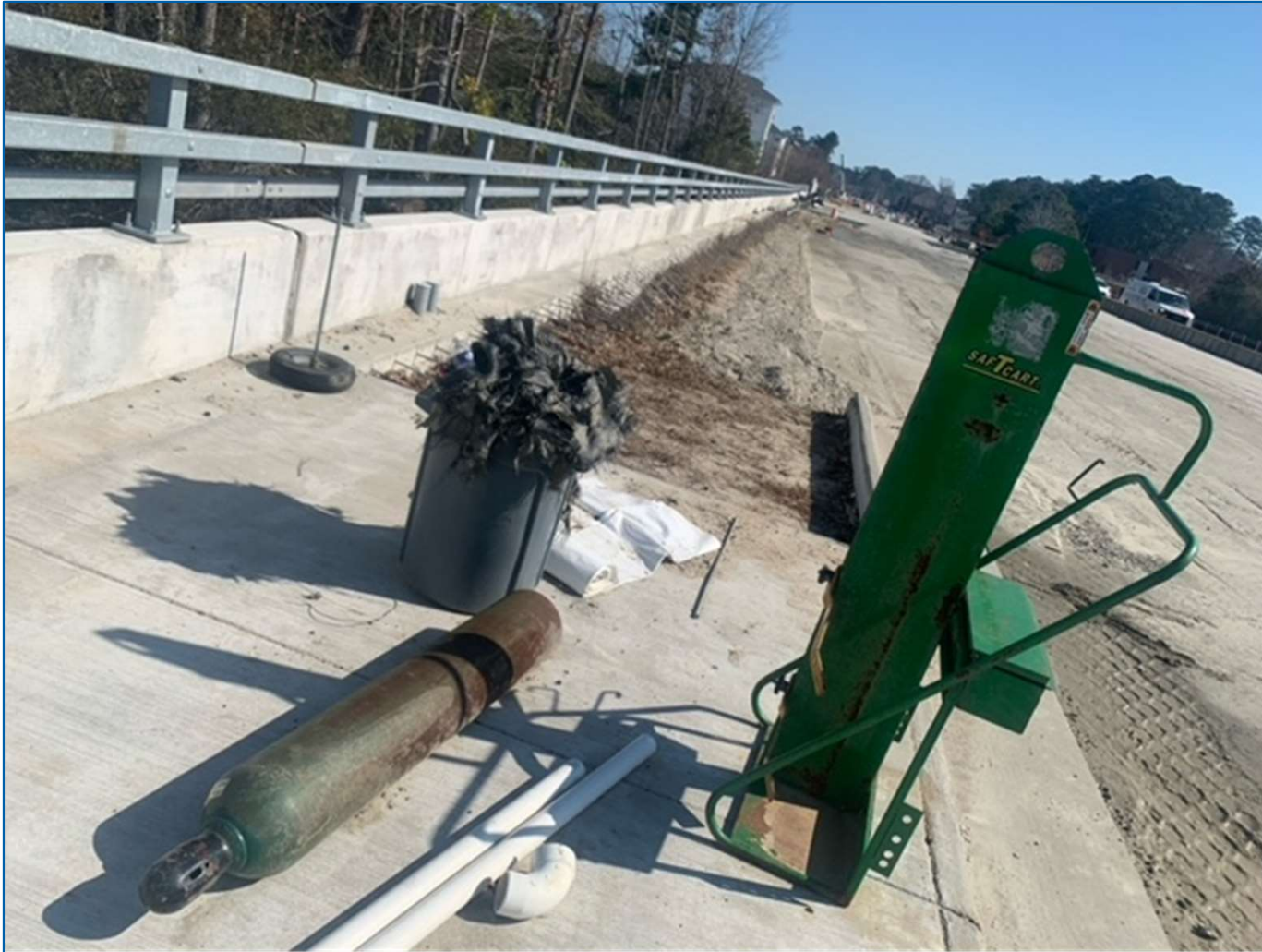
Improperly stored compressed gases
