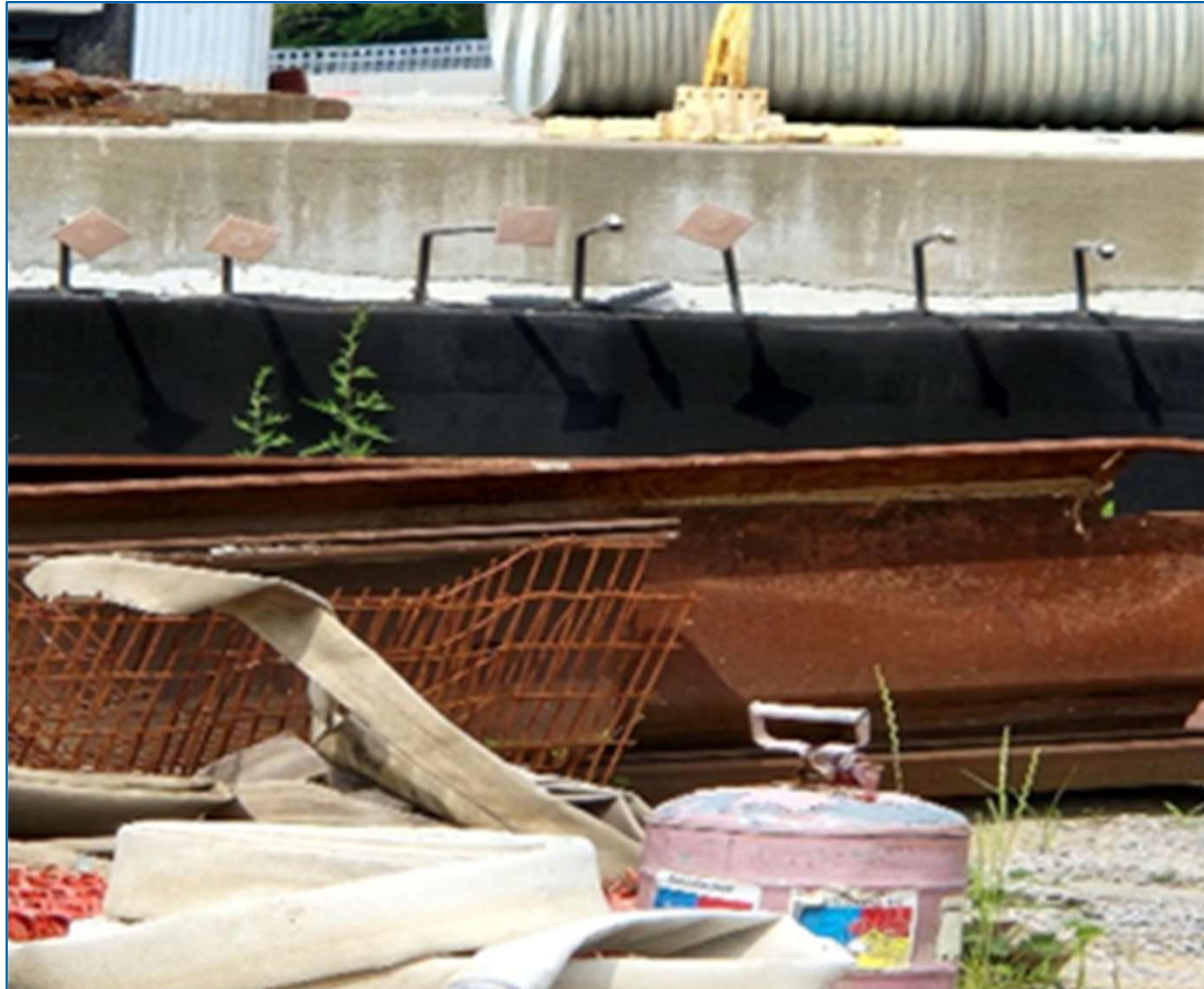
Missing protective caps on rebar
