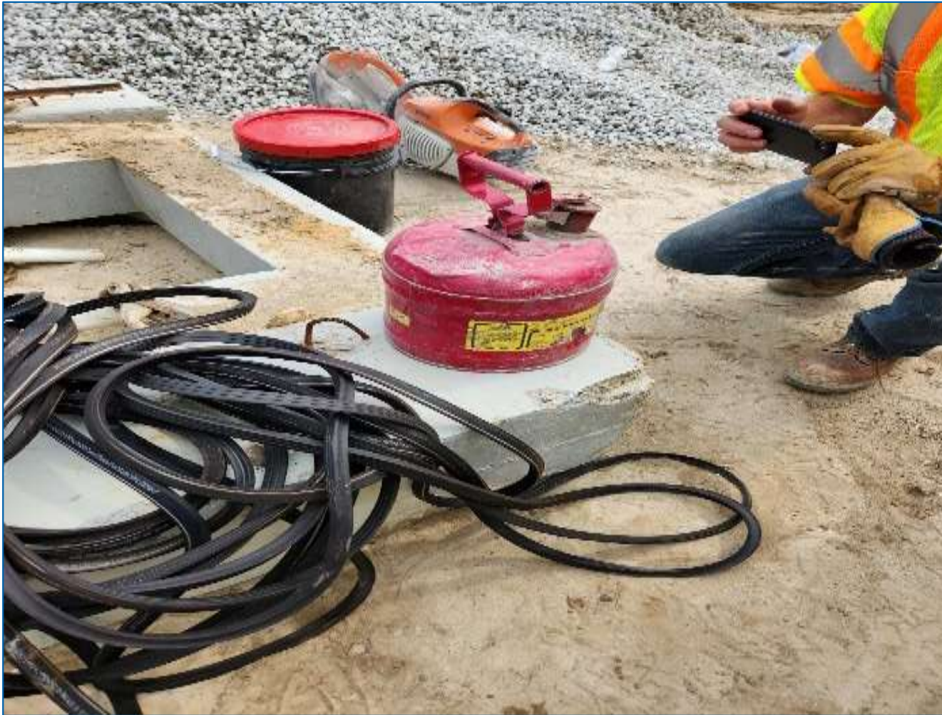
Unlabeled hazardous chemicals
