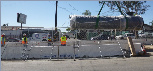
Foothill Trunkline ERDIP
