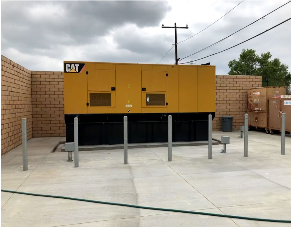
CIP # 7448 Well 10 Emergency Backup Generator
