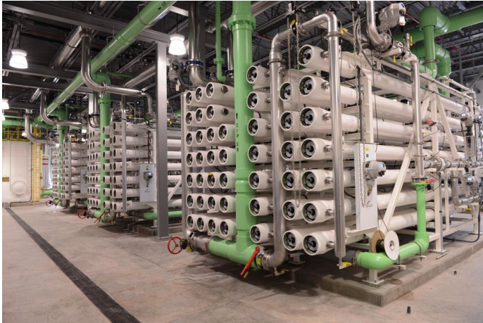
Brackish Water Desalination
