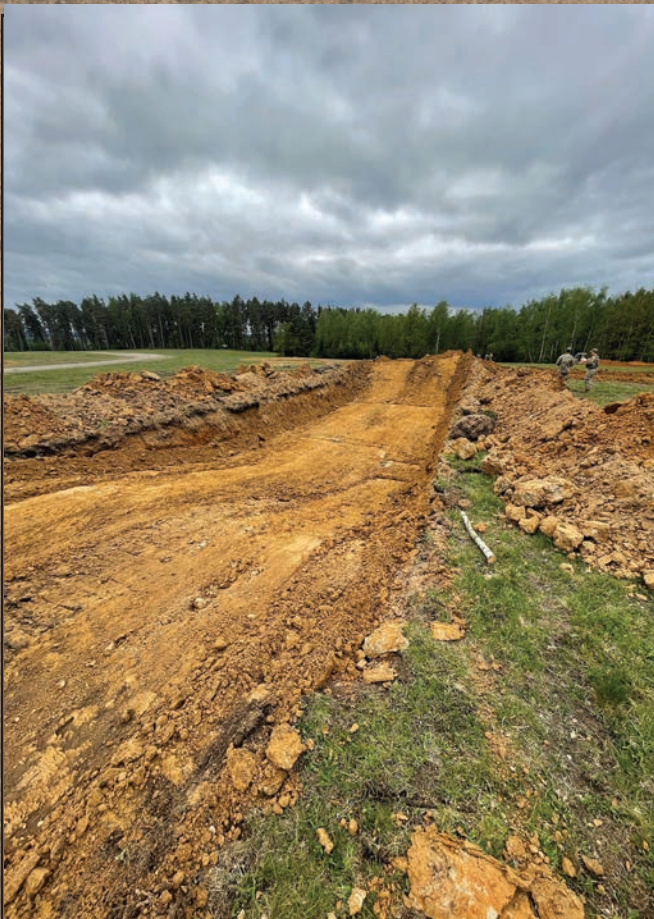
6th Section's constructed defilade position in progress. This position was built with adequate width, sub-optimal depth, and plenty of length. This version also had ramps constructed both forward and rear of the firing position as opposed to having a true berm forward of the tube.
