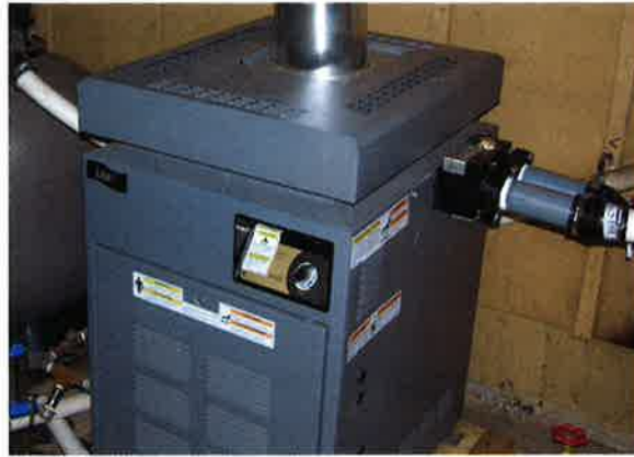
Photo 10-12. Natural gas pool heater
