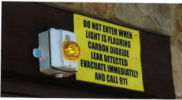
Photo 9-19. Automated systems may incorporate a variety of alarms.
