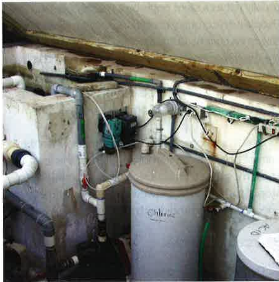
Photo 14-26. Violations of the National Electric Code, NEC 70, such as this make-shift electrical service, can lead to fires and serious injury.
