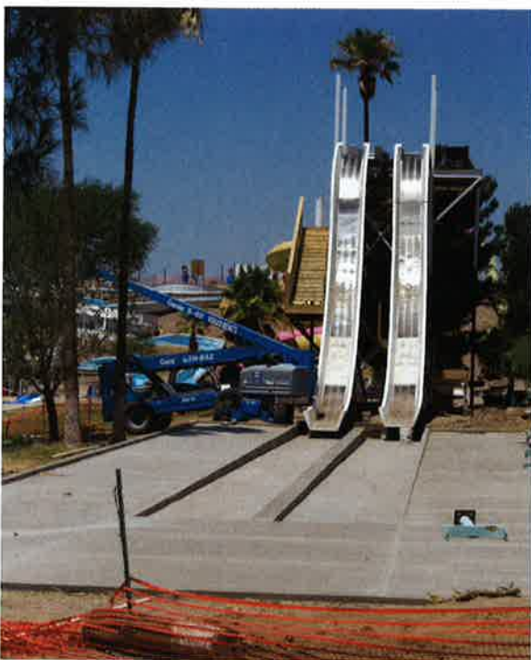
Photo 18-1. New pools and attractions require several considerations that are beyond the scope of responsibility of most pool operators.
