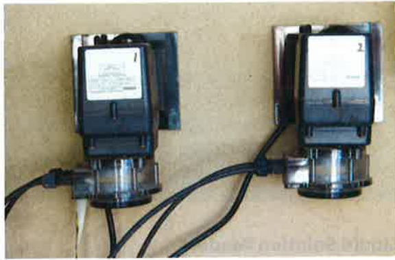
Photo 9-3. Gas chlorine systems often use a solution of soda ash dissolved into water for pH control. Positive displacement feeders introduce the solution into the circulation system.
