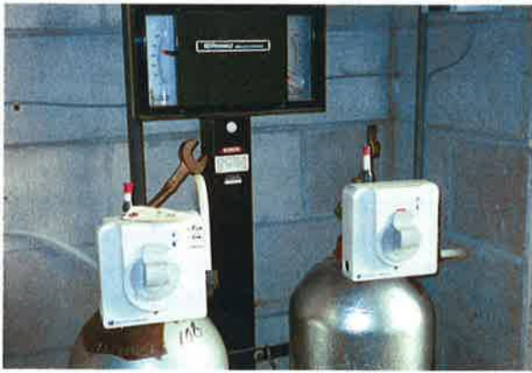
Photo 9-9. Mounted on the chlorine tank is a regulating chlorinator. A new lead gasket is always used anytime the chlorinator is removed from the cylinder.
