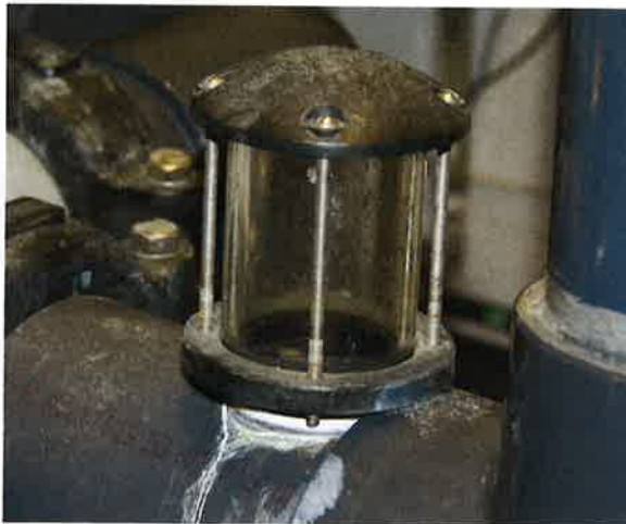
Photo 11-4. Backwash waste water is observed through a sight glass until the effluent becomes clear.
