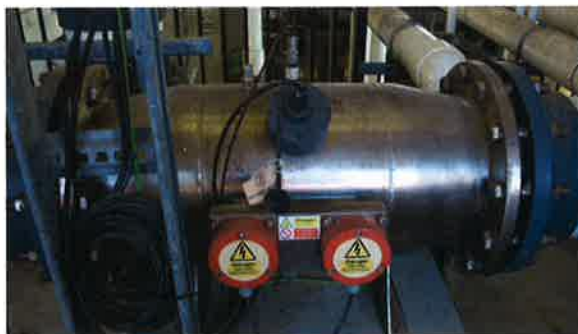
Photo 9-13. A UV system is installed so that the water flow can be bypassed so that it passes by the UV lamps.
