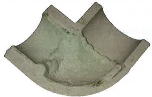
Photo 13-8. Failure to maintain proper water balance conditions may result in scale and a reduction in water flow.
