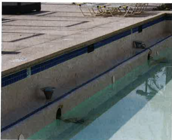
Photo 14-25. One of the most dangerous hazards to the pool and spa user is the underwater light fixture.
