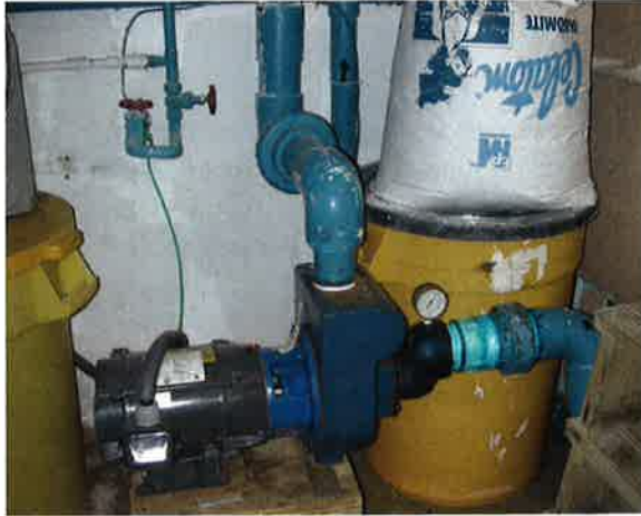
Photo 17-1. Chemicals that emit corrosive fumes and D.E. should never be stored near motors.
