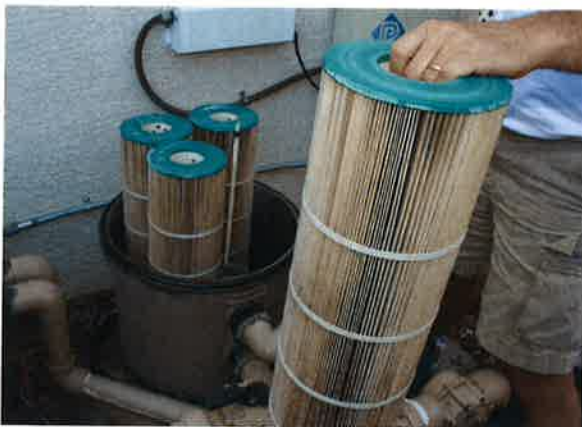
Photo 16-12. Routine maintenance, such as regular filter cleaning, is important to help ensure correct operation and extend the life of pool/spa components.
