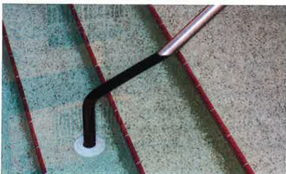
Photo 13-9. High total dissolved solids, lack of proper water balance, and perhaps improper bonding of metallic components, may result in galvanic corrosion and staining.
