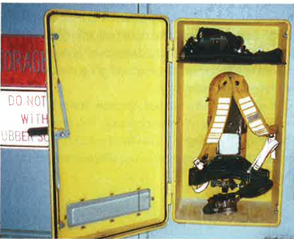
Photo 9-10. A self contained breathing apparatus should be located just outside the chlorine room.
