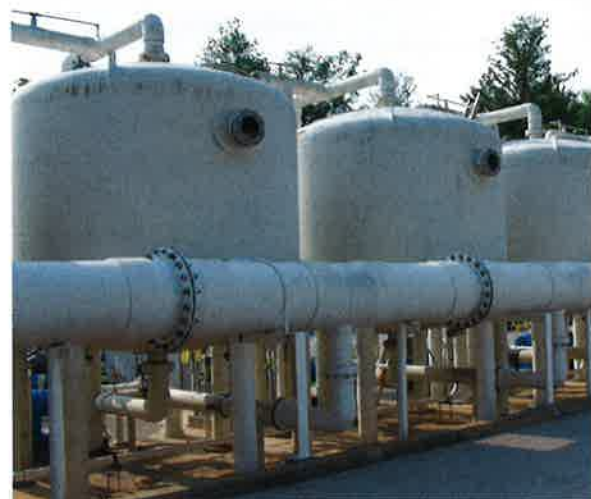
Photo 11-1. A modern high rate sand filter system
