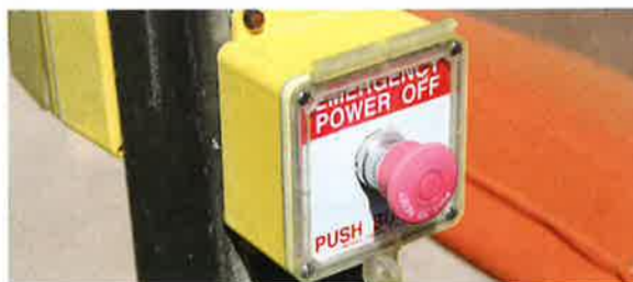
Photo 13-5. Should entrapment occur, a means of quickly shutting off the circulation system may assist in the rescue efforts.
