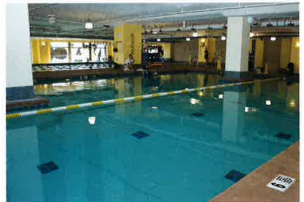
Photo 18-4. Indoor air quality is an example of a complex technical consideration requiring expert advice.
