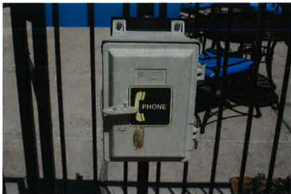
Photo 14-15. There may be no phone in the pool unless an emergency phone is installed.
