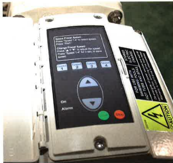
Photo 10-7. Installing variable speed motors can significantly reduce energy costs.
