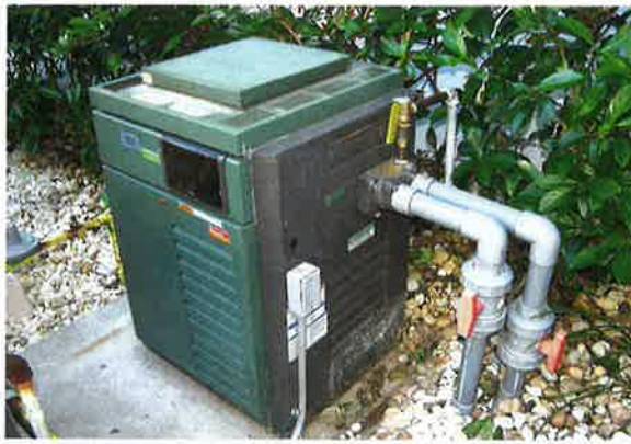
Photo 12-4. All pool/spa heaters should be positioned so their controls are not accessible to unauthorized users.
