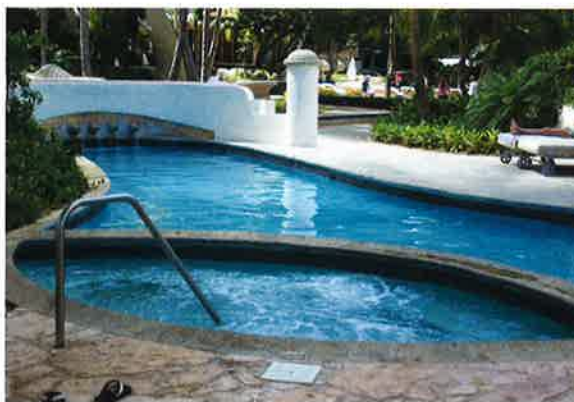
Photo 18-10. Deck repair or replacement is often part of a pool resurfacing project.
