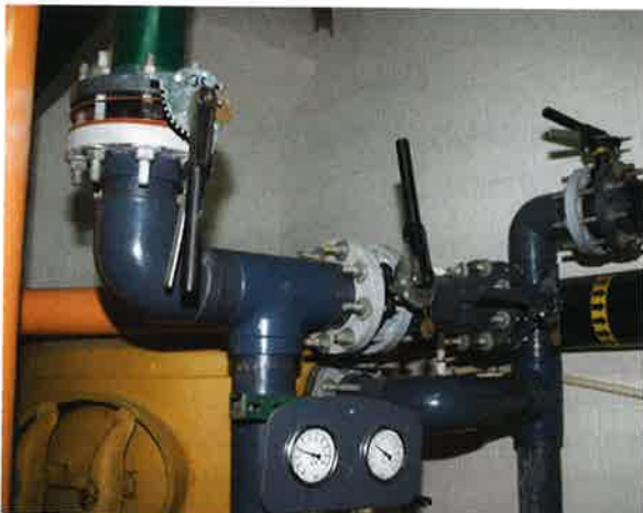
Photo 11-3. During backwash the water flow is reversed using the valve system.
