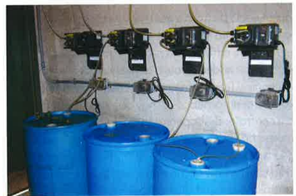
Photo 9-4. Feed pumps often have lines that can break or rupture. Care should be taken as to how these pumps are mounted above incompatible chemicals.
