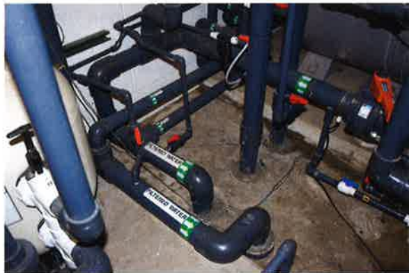
Photo 11-2. Valves should be properly tagged and a valve identification chart should be close at hand for reference by the pool operator.
