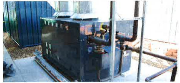
Photo 12-7. Properly sized heaters will ensure that the desired water temperature will be reached in a timely manner.
