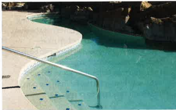
Photo 17-4. Pool water level losses greater than ¼ inch (6 mm) of water in 24 hours may be due to a leak.
