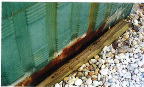
Photo 16-3. Visual inspection can spot problems, such as improper bonding, before damage becomes excessive.
