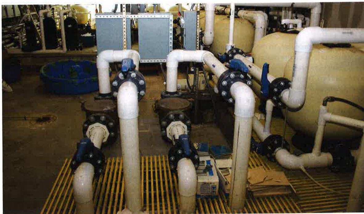
Photo 10-2. There is usually one valve to control the flow from the main drain and one valve to control the surface flow.
