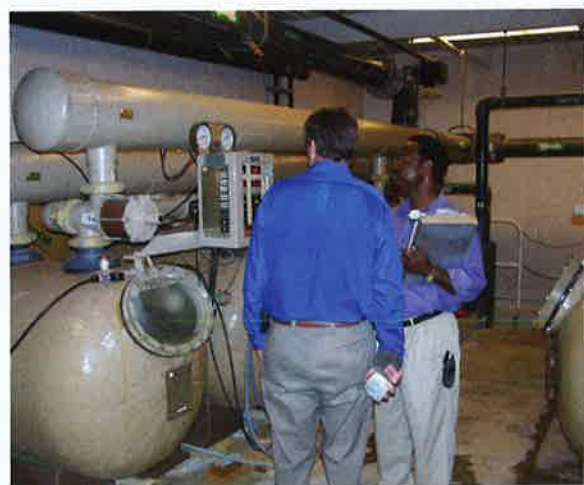
Photo 1-2. The health inspector should be considered an ally by the certified operator.
