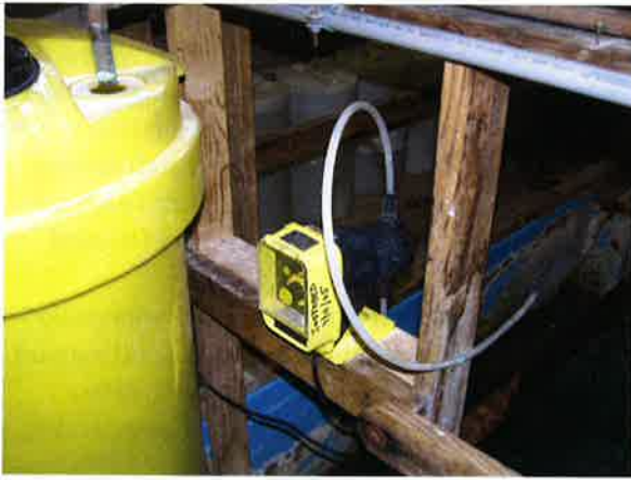
Photo 11-7. A vacuum D.E. filter slurry feed system
