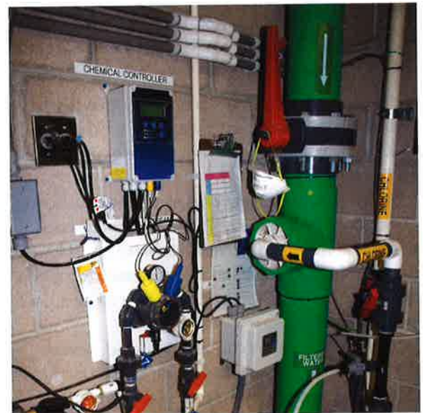
Photo 9-16. Simple ORP control systems consist of two probes (to measure pH and disinfectant), a control processor, and feed pumps to introduce chemicals.
