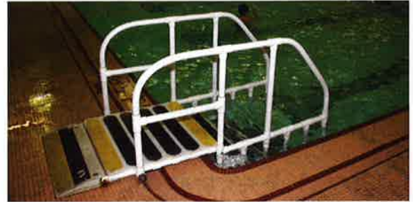
Photo 18-8. Dual handrails may not be sufficient to meet ADA guidelines.
