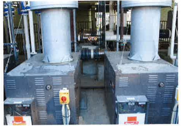
Photo 17-5. Troubleshooting gas-fired heaters must only be performed by qualified personnel.
