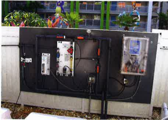
Photo 18-5. Automatic chemical feed control can be made part of any modernization project.
