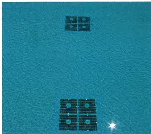
Photo C1-2: Dual main drains more than 3 feet apart
