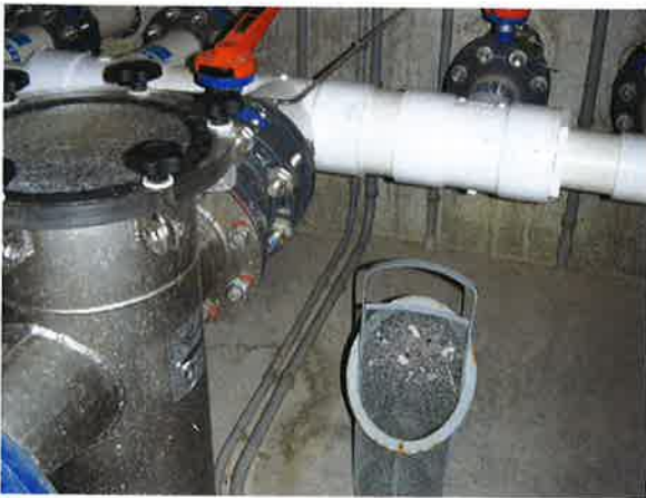
Photo 17-3. Clogged hair and lint strainers may be a blockage in the suction line, causing the motor to be noisy.
