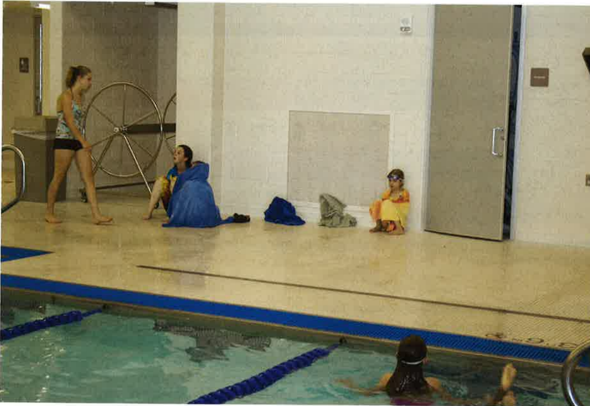
Photo 12-9. Ventilation system design and operation is important to achieve good air quality at indoor aquatic facilities. Low level air returns help to carry away gasses evaporating from the water.
