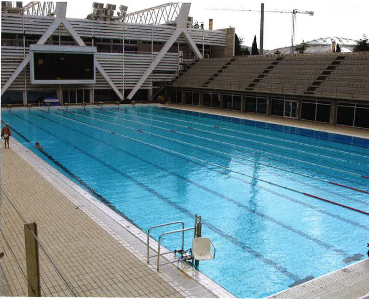
Photo 11-9. Turnover rates and flow rates must be carefully considered based on the design size of the pool.
