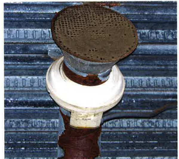
Photo 16-7. Preventative maintenance may also include making sure that the vent covers in the pump room are kept clean to ensure adequate ventilation.
