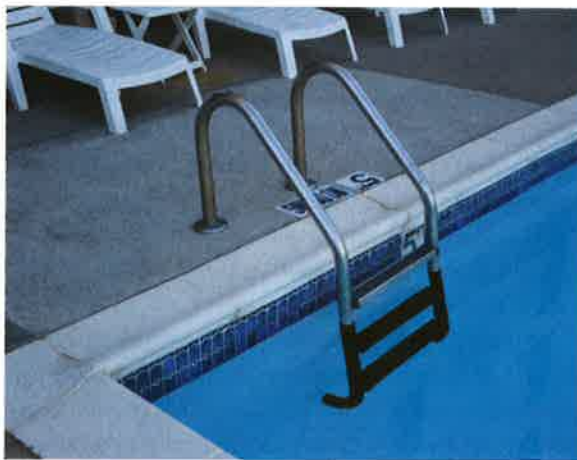
Photo 6-2. An example of galvanic corrosion. Copper staining on a stainless steel surface as a result of high TDS and improper bonding and grounding.
