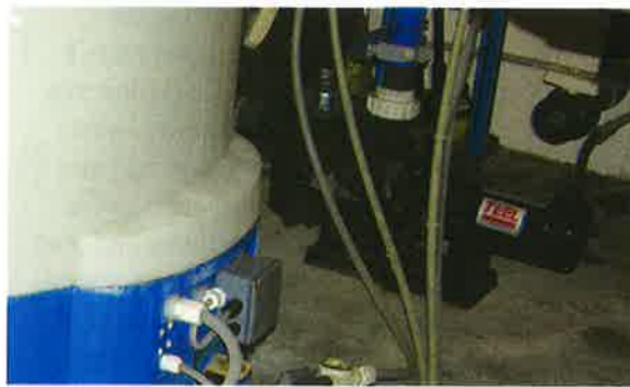
Photo 9-7. Booster pumps are often used to introduce chemicals into the circulation line.
