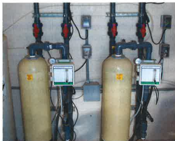
Photo 9-8. Most gas feed systems rely on the venturi principle to mix the gas into the circulation water flow so that the gas is properly dissolved.
