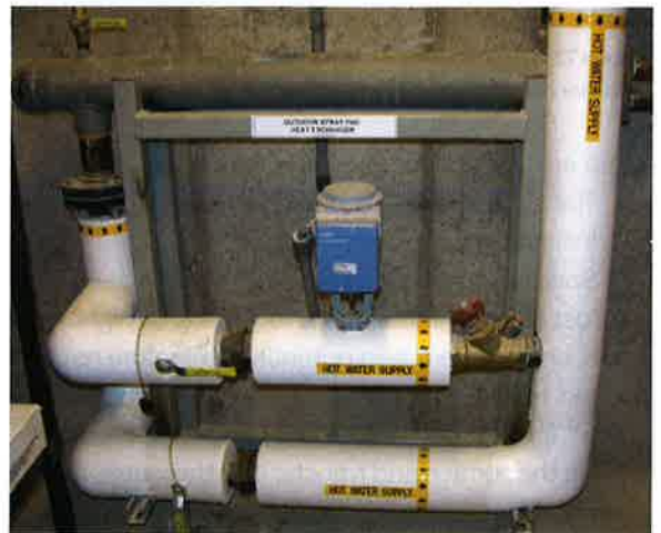
Photo 12-5. Heat exchangers utilize the existing hot water supply of a building to heat the swimming pool water.
