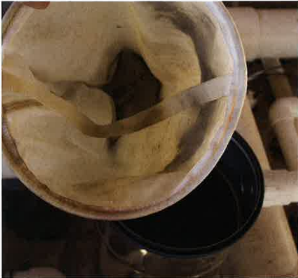
Photo 10-11. Separation Tanks have internal bags to collect the spent D.E. powder.
