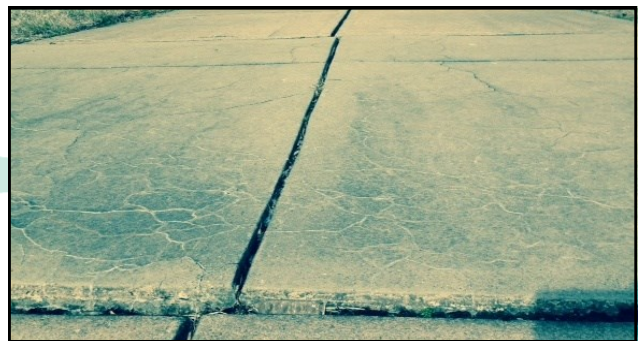
ASR Cracking and Expansion in Sidewalk
