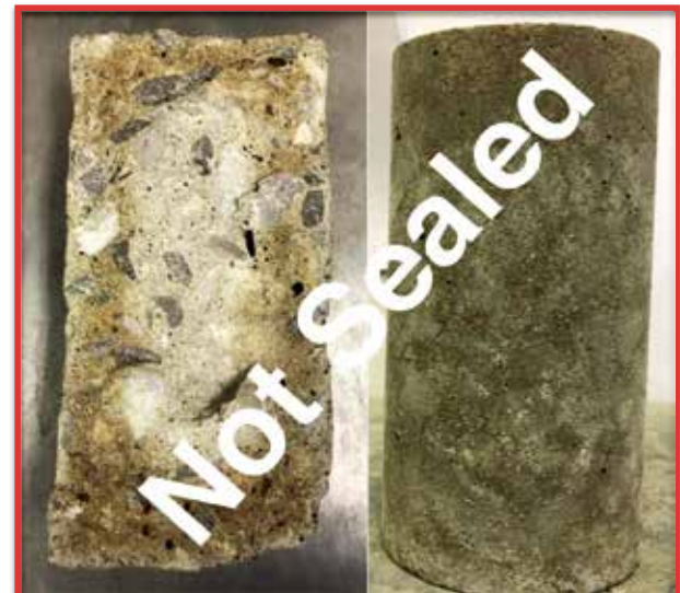
Normal Concrete WITHOUT A SEALER. Notice the deicer has penetrated deep into the concrete.
