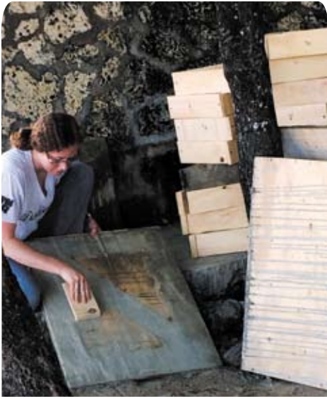
CIM senior, Katie Poss, sands concrete off a used form for reuse.
