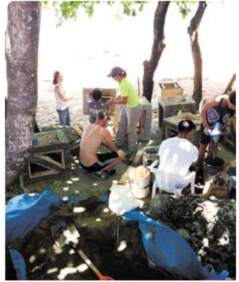
Students work on the beach to prepare forms and mix concrete for use.
