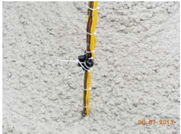
Figure 6: Close-up of Temperature Sensors In-place
