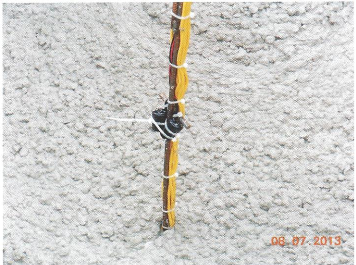
Figure 6: Close-up of Temperature Sensors In-place
