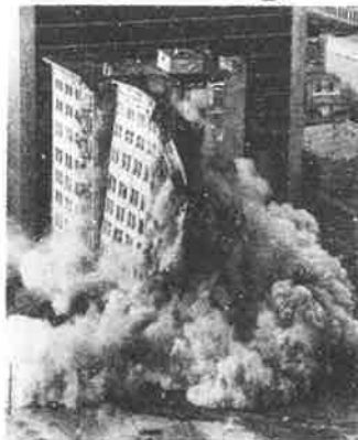
2 250 pounds of explosives split the 10-story structure in halves early Sunday with two soft booms.
