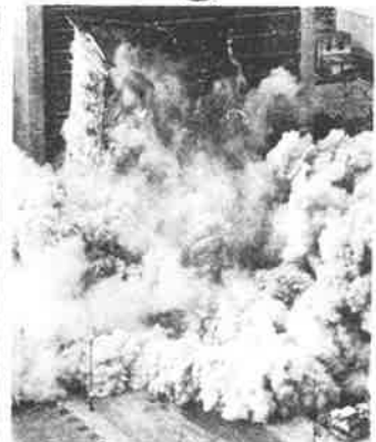
3 Taking only 6 seconds to destroy the building, the implosion did not damage surrounding structures.
