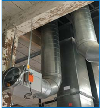
Fire smoke damper installed on 2nd floor.
