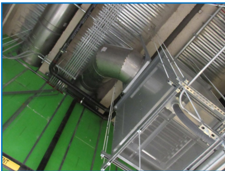
8th floor mechanical equipment muffer.
