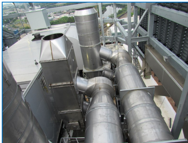
Roof view of boilers that go all the way to the basement.
