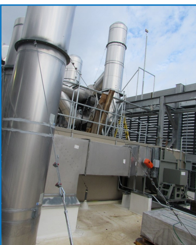
Generator exhaust from that starts on 8th floor to roof.
