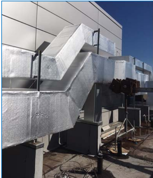
Roof duct for eru1, supplying air to the tower for floors 3-13.
