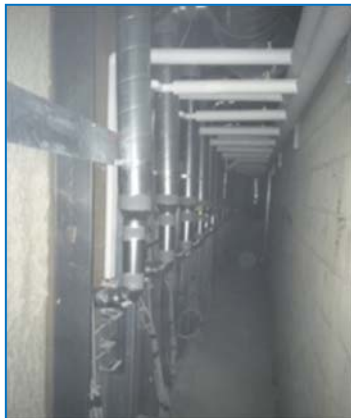
Dryer duct bank of 17 units
