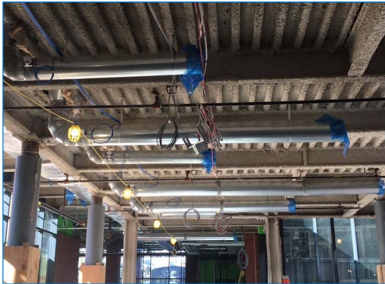
Ductwork in the new student dining room.
