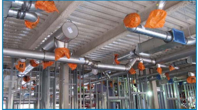
Fully installed duct in one of the lab areas on Second Floor.
