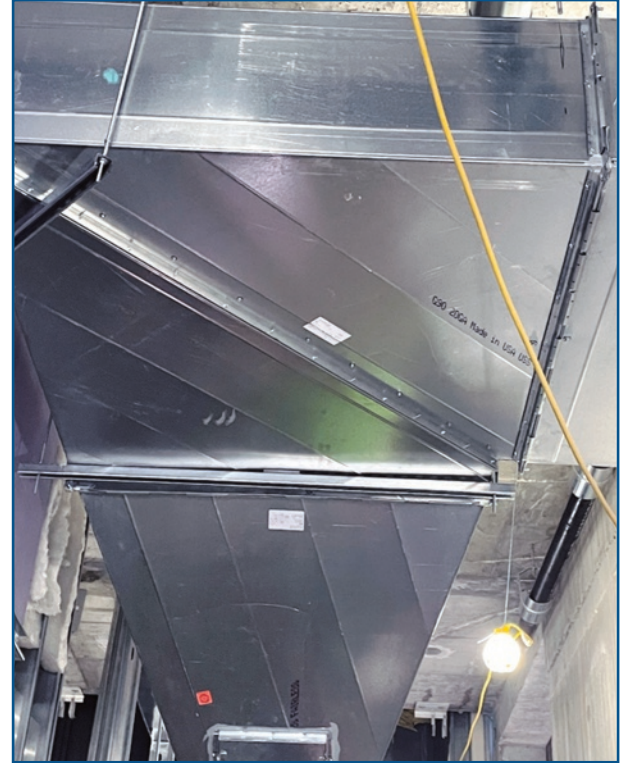
Outside riser on 32nd floor.
