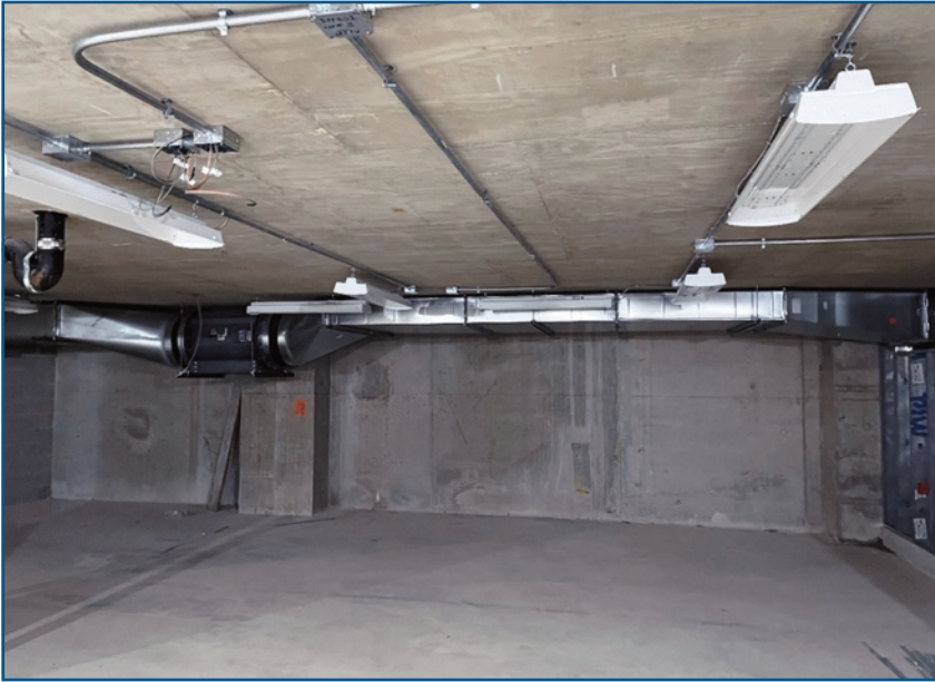
Garage units that will exhaust all car fumes out of the building.
