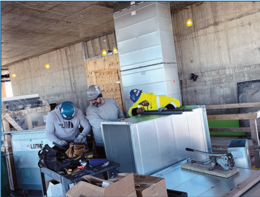
(L-R) Brent Long, Dave Harris, and Mike Sullivan are preparing units outside air 2 and exhaust air 13 on the 31st floor.
