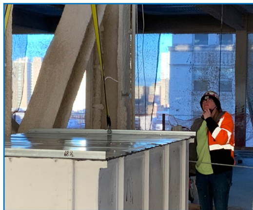
Marlana Jost communicates with crane operator on lowering second large piece of ductwork.
