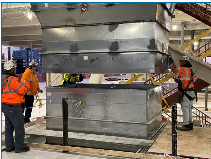
Dan Greenwald communicates with crane operator lowering ductwork. Mo Shuster helps guide the ductwork to make connections.
