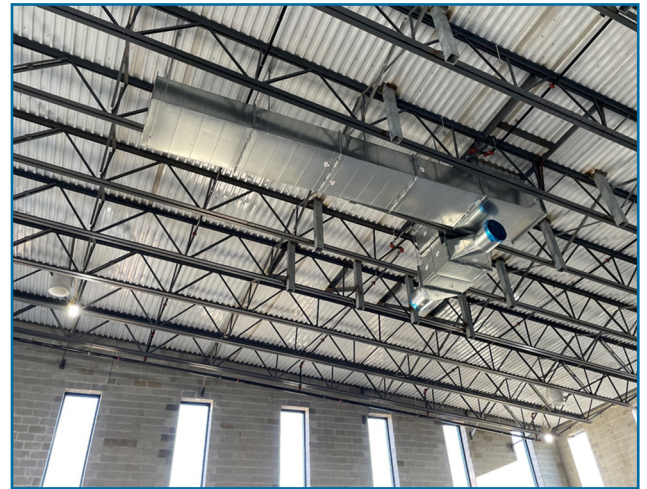
Roof-top-unit in gymnasium.
