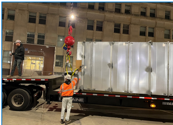
Mo Shuster (orange safety vest) and Dennis Pollock are prepping for ductwork to be hoisted.
