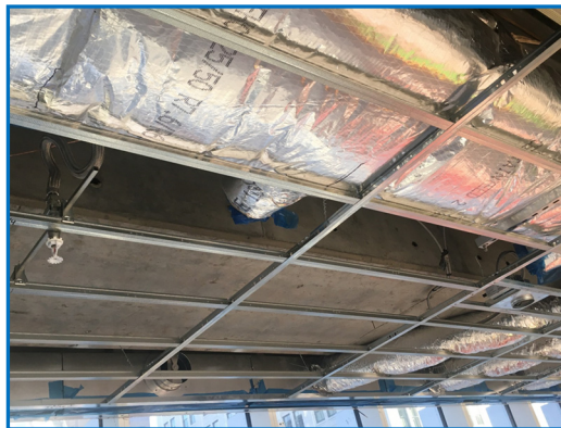
Continuous plenums with cable operating dampers (COD) around the pool area.
