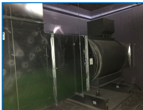
Exhaust fans installed in the cellar.
