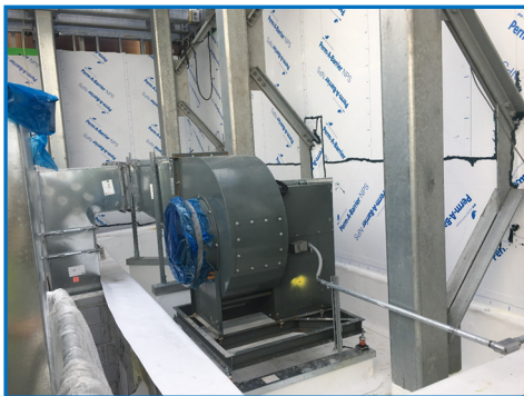
47th floor stair pressurization fans.
