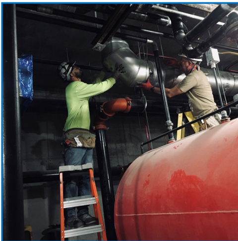
Brian Buchanan (left) and Matt Cahill (right) are in the pump room area connecting an elbow duct piece.
