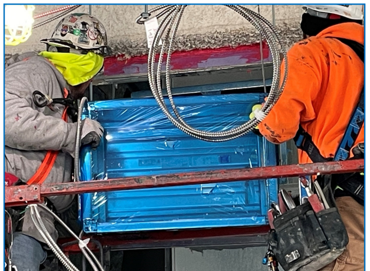
Dave Vuich and Ron Correlli installing riser deck fire smoke damper on 5th floor.
