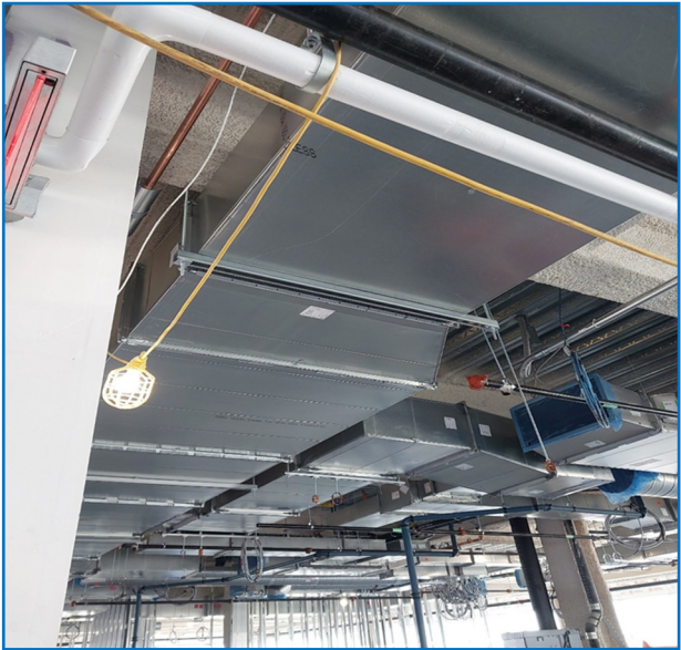
One uCity Ductwork
