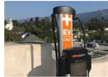
EV charger at Granada lot
