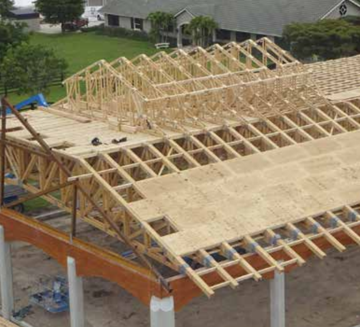
Figure 1. The box beam trusses were piggybacked and included windows located within the lower portion of the cap truss.
