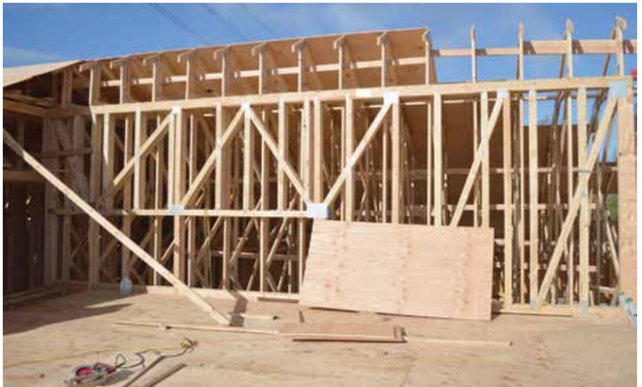
Figure 5 and 6. The Truss Company's team designed an intricate 4-ply girder truss, over 15 ft. tall with a cap truss, for the area next to the attic and mechanical platform.
