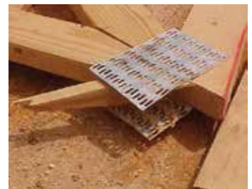
Figure 3. Improper handling of trusses can result in permanent damage.
