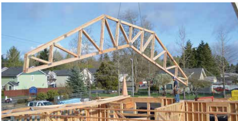
Figure 4. Installation of a scissor truss. With a cap truss installed, many of the project’s scissor trusses were over 15 ft. tall.
