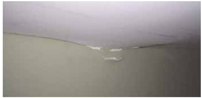
Figure 1. A wood bearing failure is not catastrophic; however, finish damage, cracks, and sagging result from local wood crushing
