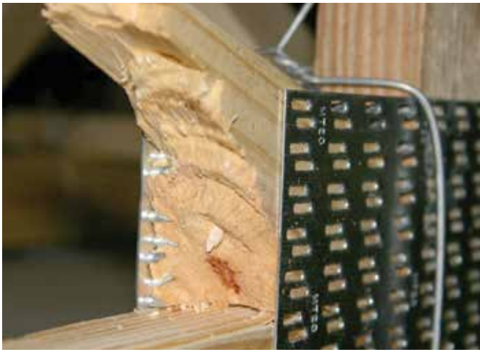
This was the first brash tension web failure in the lower right truss in the picture above. SBCRI staff tested this #1 SP web in bending to define its properties.
