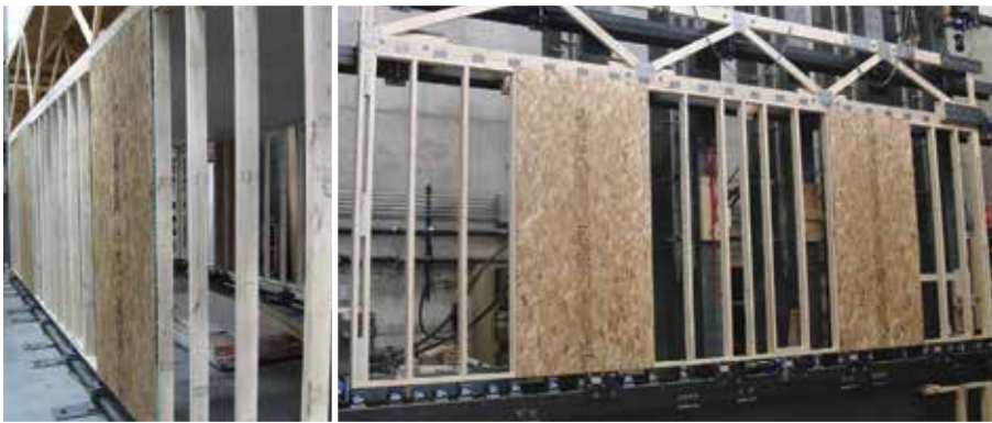
Figure 3. Isolated 4x8 Wall Testing: The results from the 12' x 30' building tests were compared to the new SBCRI lateral wall station with truss framing tests to ensure they produce similar results.
