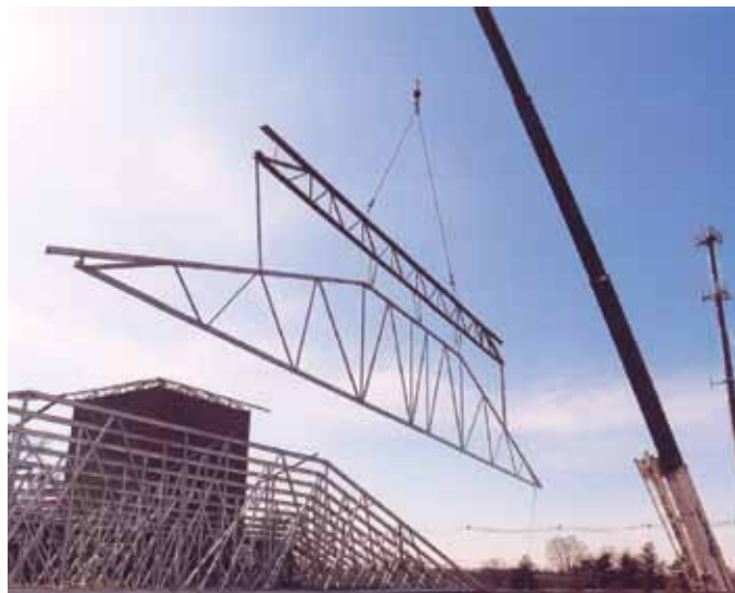
Photo 1. Example using a spreader bar to lift cold-formed steel trusses greater than 30' in length.
