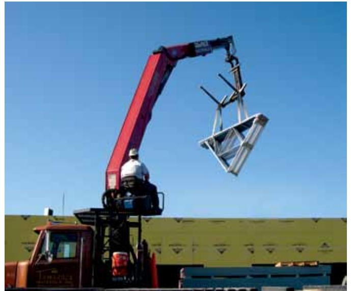
Photos 2 & 3. Bundles of metal plate connected wood and cold-formed steel trusses being hoisted onto a structure.
