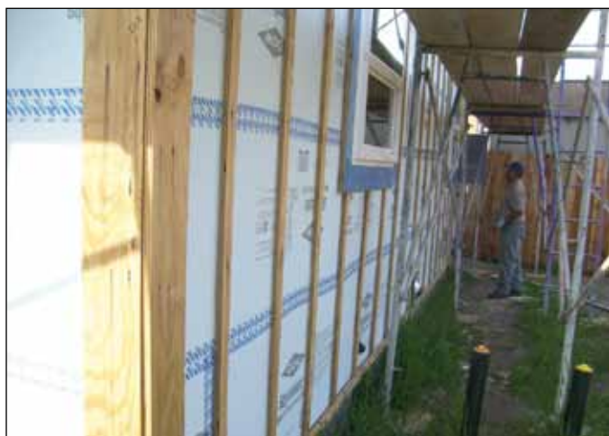
Photos 6. Siding installation posed a bit of a challenge, which was solved by adding extra furring strips to attach the siding.
