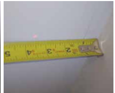
Photo 2. Smaller sheet rock crack resulting from insufficient bearing area.
