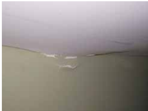
Photo 1. Significant sheet rock bulging and cracks resulting from insufficient bearing area.
