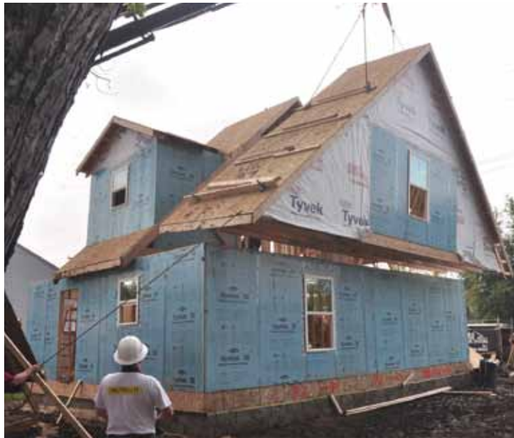
Photo 4. After the first-floor walls are set, the roof sections were craned above the top plate.
