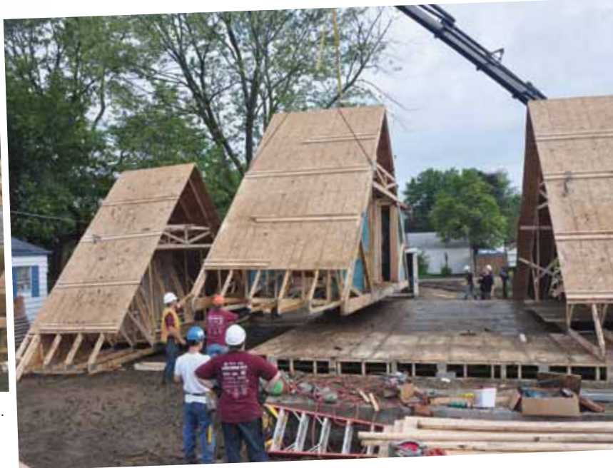
Photo 2. The second floor was then lifted off in three sections and set aside.
