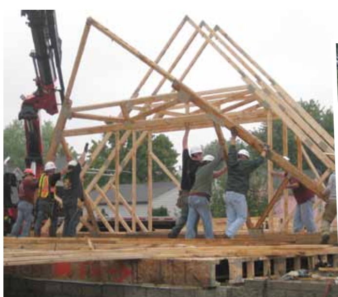
Photo 1. The entire second floor was framed on top of the first-floor decking.
