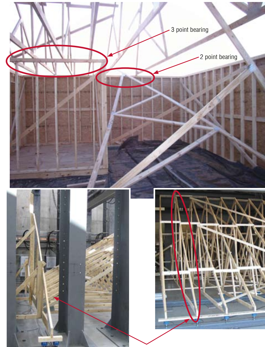
The A2 truss that broke in the field
