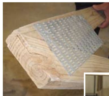
Damage to the actual truss on the jobsite. It shows splitting at the end of the bottom chord.
