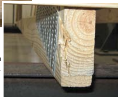
The end of truss A2 used in SBCRI shows splitting.
