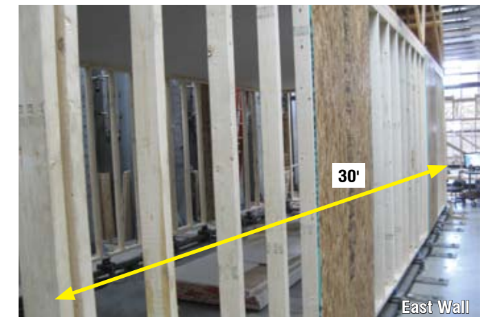
Photo 3. For SBCRI's 3/8" wood structural panel (WSP) test, the braced wall panel consisted of two 4x8 sheets (8' of bracing) and the braced wall line was 30' long.
