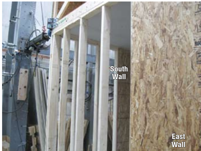
Photo 7. As defined by the IRC, there was no OSB corner return deployed, and the end walls had a single sheet of OSB in the center of the 12' wide wall on both the exterior and interior faces. This was intended to provide end wall bracing support only and did not affect the braced wall line performance.
