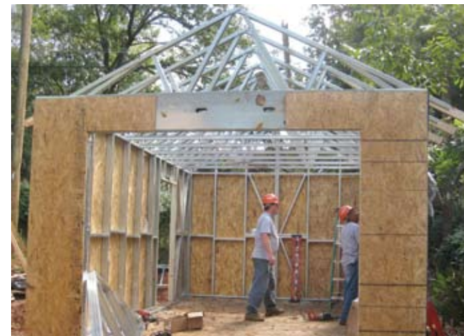
Volunteers from NUCONSTEEL framed the family's garage with cold-formed steel on Day 2.
