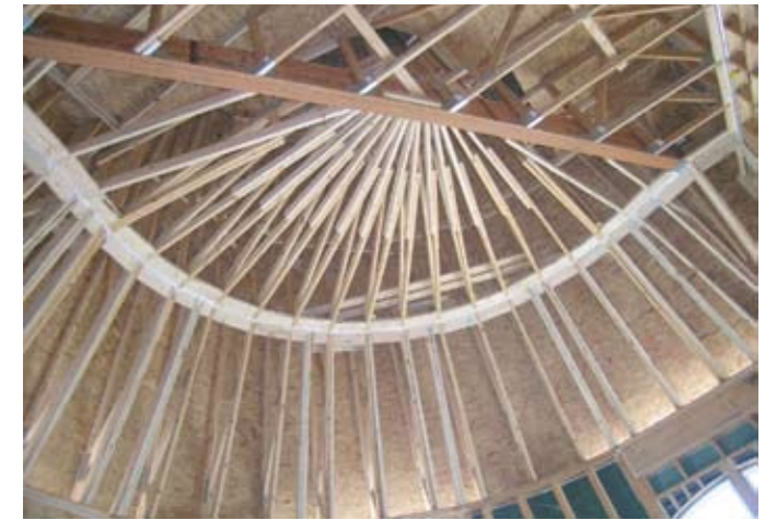
The tower is framed with high-heeled scissor trusses, creating a true conical roof shape. Scabs added to the sides of many truss bottom chords create an alternating straight and curved shape at the top of the wall. This makes way for the transition to a true continuous circle for the tower. A total of 15 trusses with a 28/12 pitch create a “fan effect,” said Kolosky. The trusses tie into the angled beam (top).
