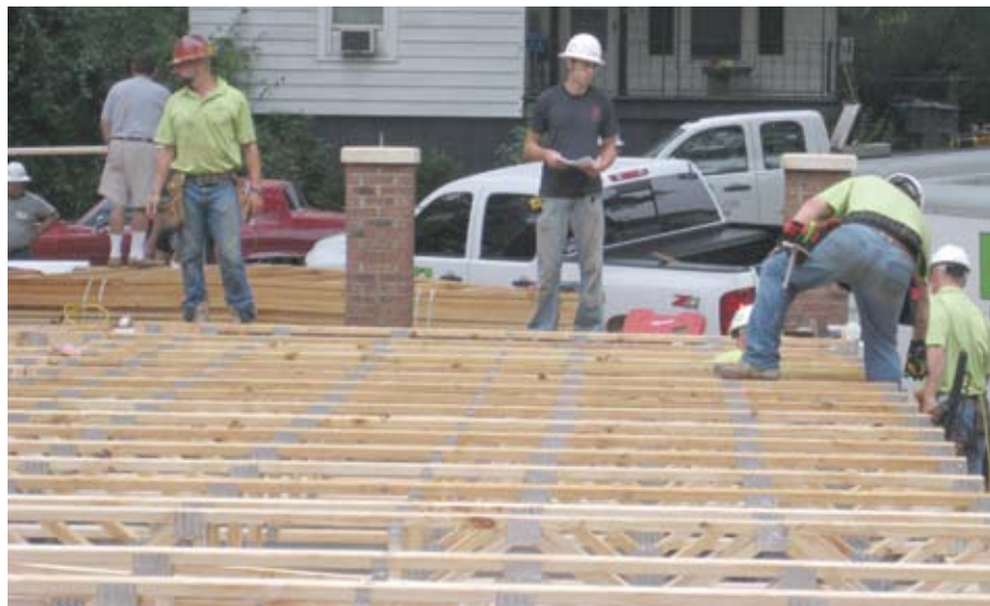
Volunteers from Capital Structures put the finishing touches on the floor trusses.
