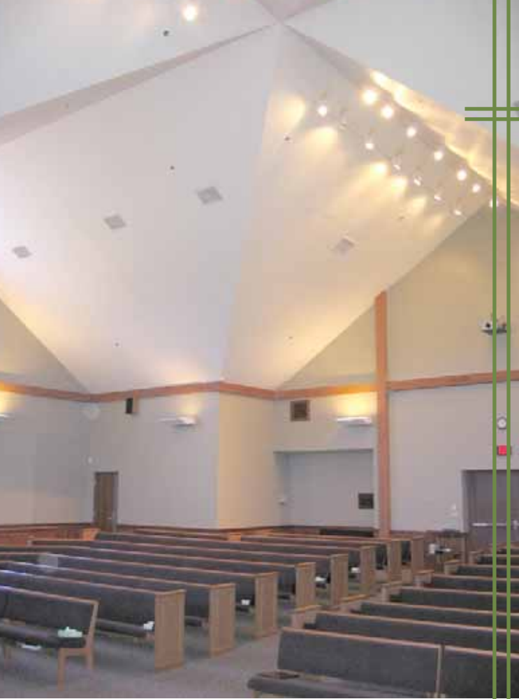
Photo 2. For aesthetic purposes, the glulam beams are all exposed on the inside of the finished structure
