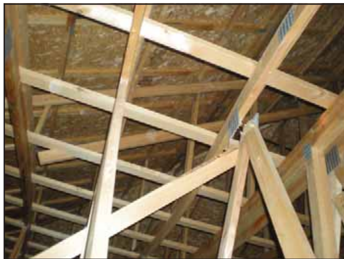
Photo 3. Broken top chord joint in one of the trusses. The diagonal brace attached to the web at this joint kept the webs from moving laterally with the top chord.
