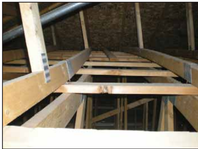
Photo 2. Bottom chords of "cap" trusses are deformed to same general shape as the top chords of the supporting trusses.
