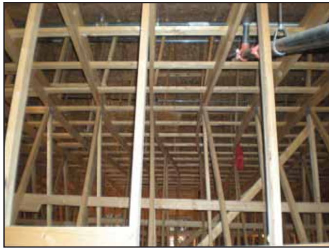
Photo 1. Buckled top chords of supporting trusses in piggyback system resulting from a failure to install diagonal bracing in top chord plane.
