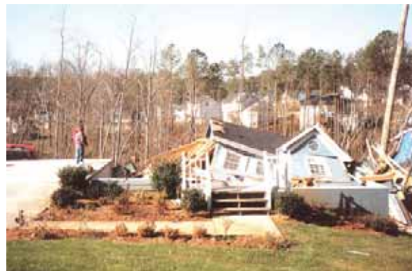
This dramatic collapse photo revealed incorrect framing practices.
