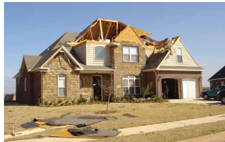
Tornado damage exposed framing issues that revealed structural defects in this home.
