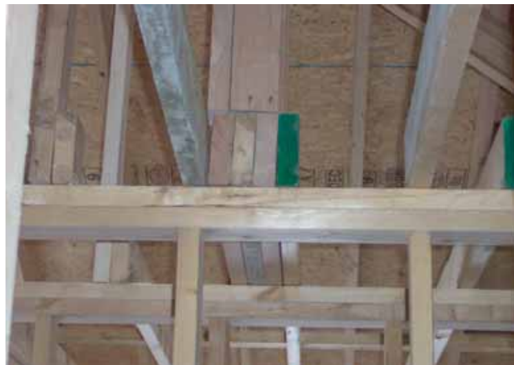
Spradlin says examples of poor framing practices can be found in his market. For example, in this photo, a 4-ply beam bearing on a wall has no studs under it to transfer the load to the floor below.
