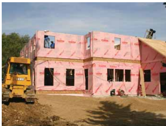
Walls for the Richco project were set ahead of schedule, speeding up framing overall and allowing designers more time to work on the interior of the house.
