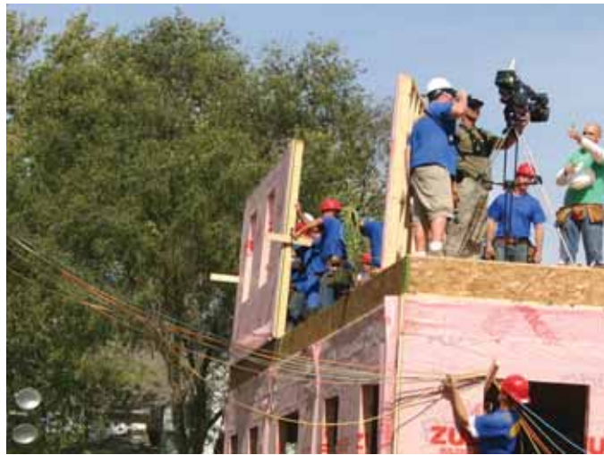
Work continued at a steady pace for framers on the Richco site, while the show's cast filmed segments.
