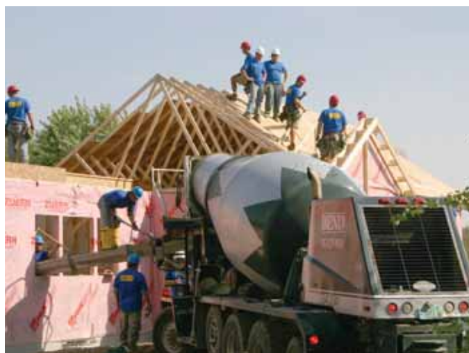
Coordination is key for any Extreme build. At the Richco site, sheathing was applied to the garage roof while concrete was poured for the basement below.
