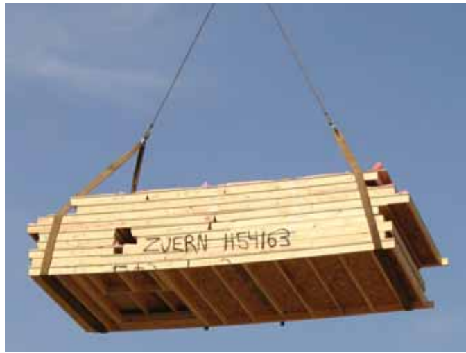
Wall panels were hoisted to the second floor of the building on the Richco site.
