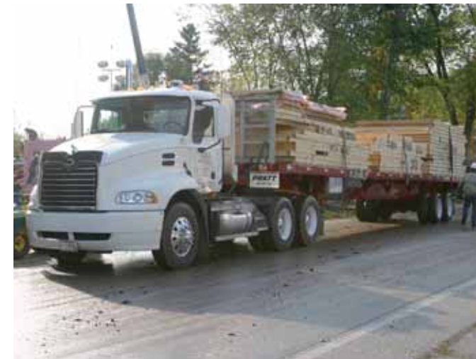
Coordinating deliveries was especially important for the Richco project because the site was located on a small city street, so trucks had to quickly unload materials and move to make room for the next delivery.
