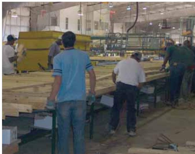
Lumber is placed on a table in preparation for the headers to be nailed.
