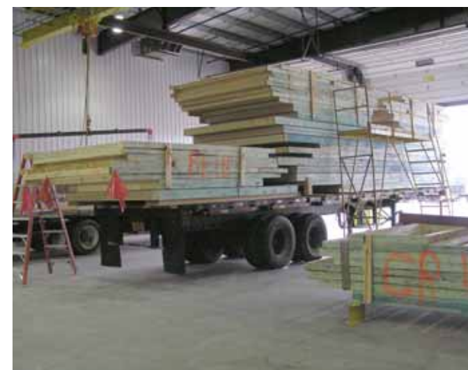
Walls are loaded on the delivery truck so framers can work in sequence, eliminating the need for double handling.
