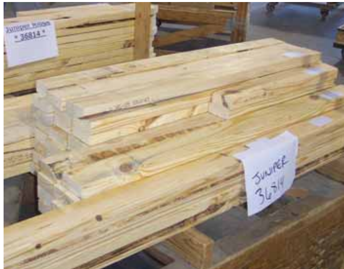
Webs are neatly stacked on a cart according to their placement in the truss and labeled with the job title and number.
