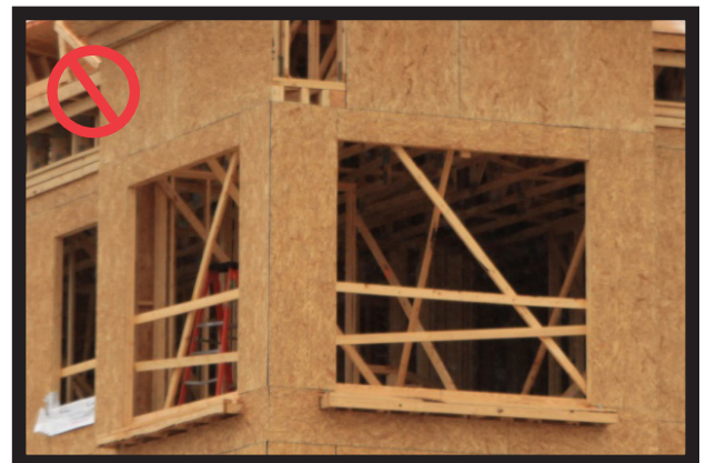
Poorly built guardrails draw attention to other safety concerns.
