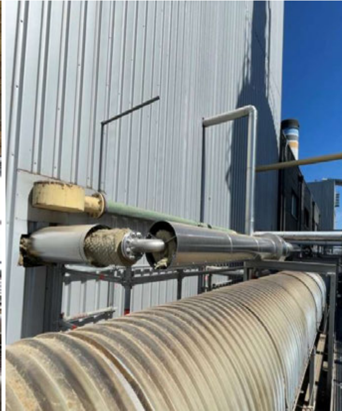
Pipe to hot-gas generator
