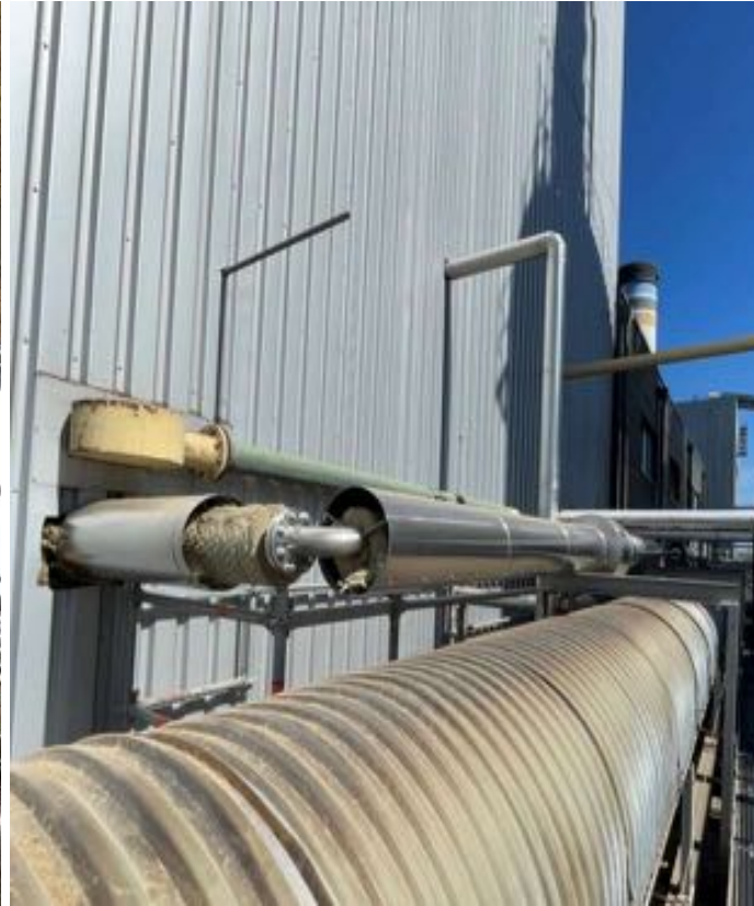
Pipe to hot-gas generator
