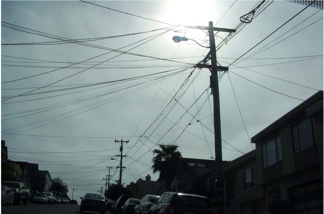
Figure 2: Crowded Utility Pole Line in Bayview
