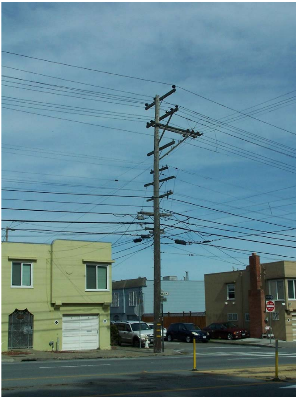
Figure 3: Utility Pole Requiring Make-Ready in Excelsior
