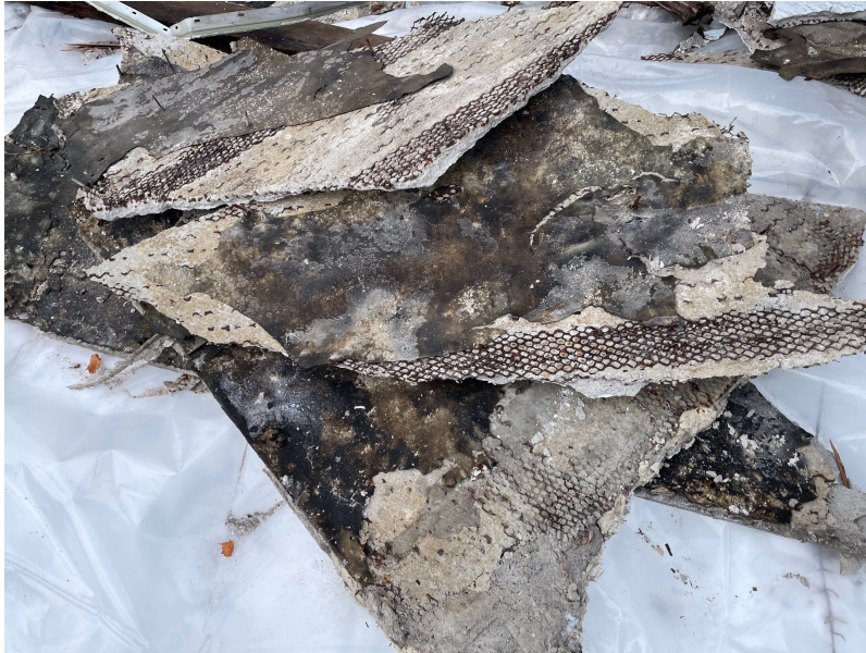
Removing the existing wall finishes revealed concealed mold and moisture damage.
