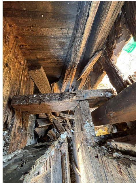
Demolition exposed compromised wood framing hidden within the existing structure.
