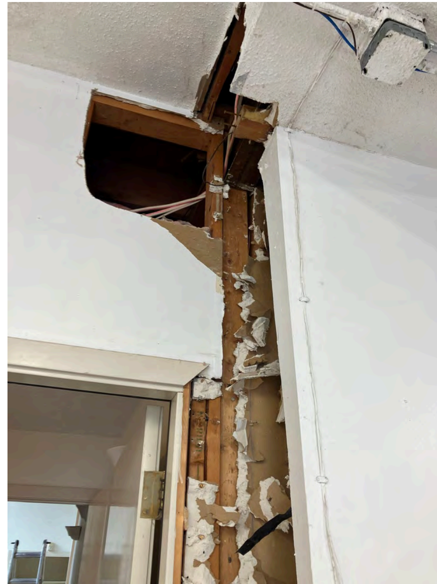
Old support configuration leading into mudroom.
