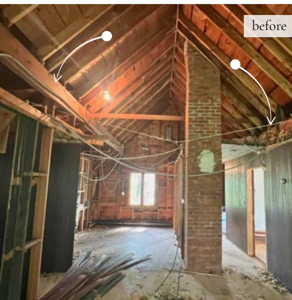
Roofs bears down on these supporting walls
