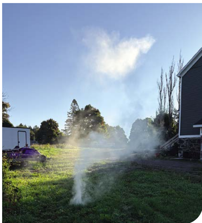
Smoke testing for I&I, smoke rising from a broken sewer lead.
