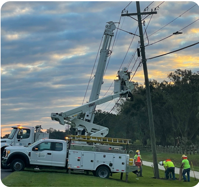
The MMUA-led mutual aid crews help repair lines and clean up debris in Florida following Hurricane Ian.
