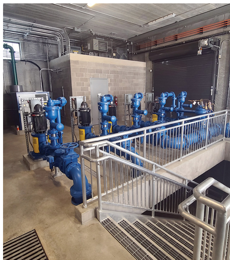
The pump room in the new plant.
