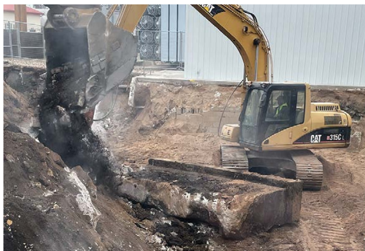
The removal of the old steam plant's footing was necessary to put in the foundation for the new generation plant building.
