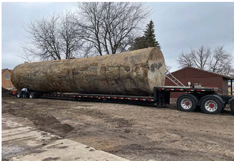
The outgoing 50,000-gallon underground fuel tank.
