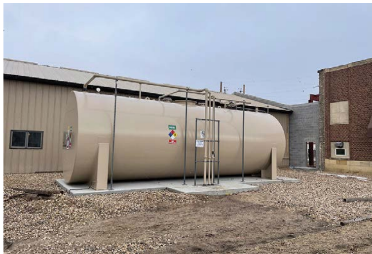
The new 20,000-gallon fuel tank.
